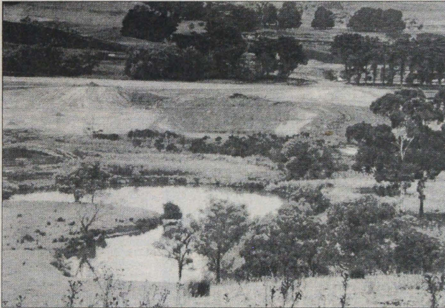
Earthworks for a golf course near Mt Lofty. Is this the future for the Green Wedge?
