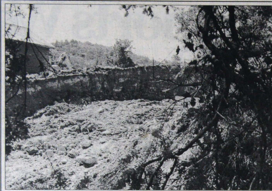
Men at work: excavations for the driveway to the carpark behind the seven new shops in Yarra Street. (Picture by Jan Tindale)
