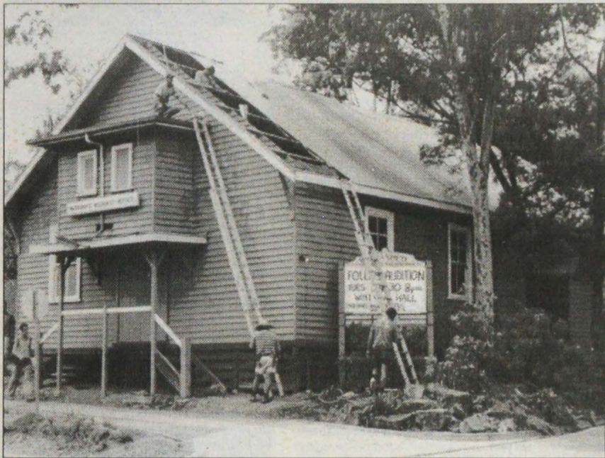
A new hat for the hall: Warrandyte Arts Association have been raising money to replace the roof on the Mechanics Institute Hall for years. Recently, Manningham council topped up their fund with a generous grant. Diary photographer Jan Tindale caught these men at work, putting the finishing touches to the new roof, late last month.
