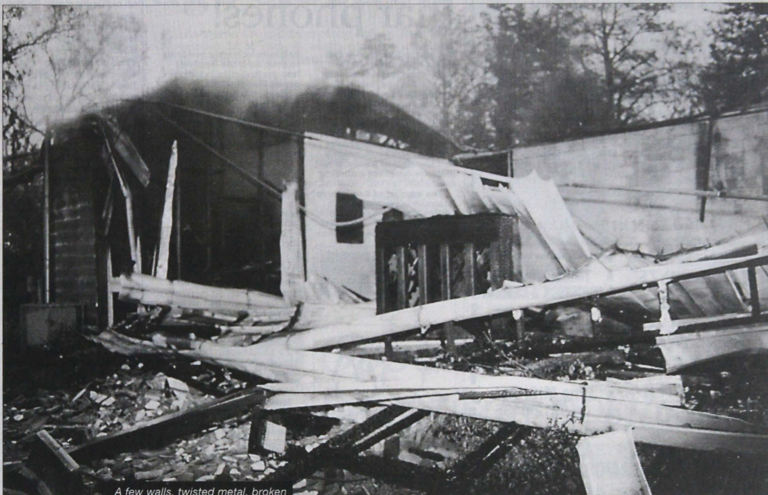
A few walls, twisted metal, broken bricks and ashes: all that remains of the North Warrandyte Community Centre. (Pictures by Sandy Burgoyne)
