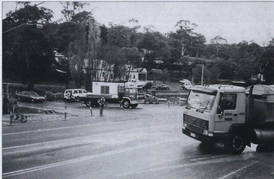
Men at work: new roundabout at Jumping Creek Road intersection is underway. (Picture by Jan Tindale)
