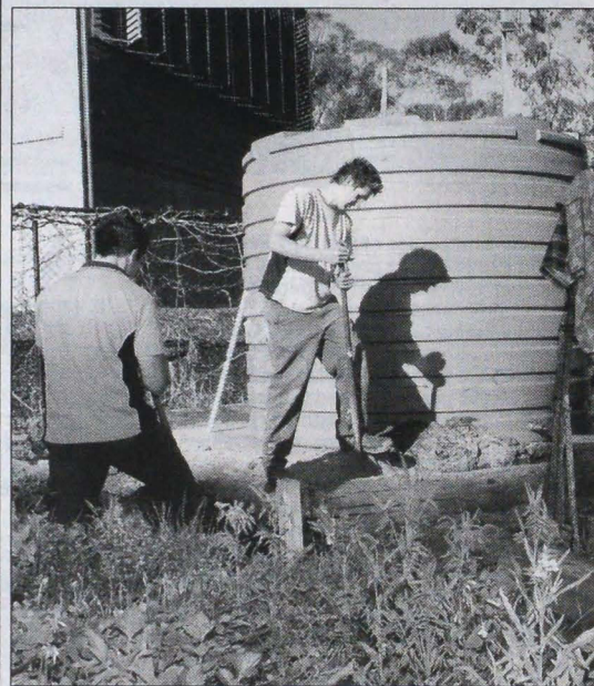
The right connections: plumbers install the rainwater tank at the Warrandyte Community Garden. (Picture by Sandy Burgoyne)
