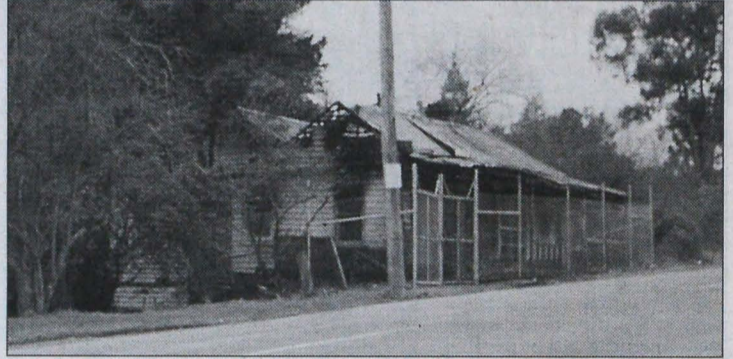
The old post office following the fire, which many locals believe was deliberately lit.
