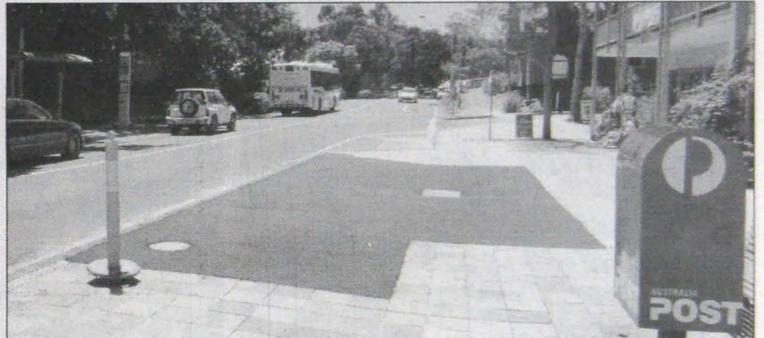
3 A bitumen seal makes unfinished work 'safe'.
