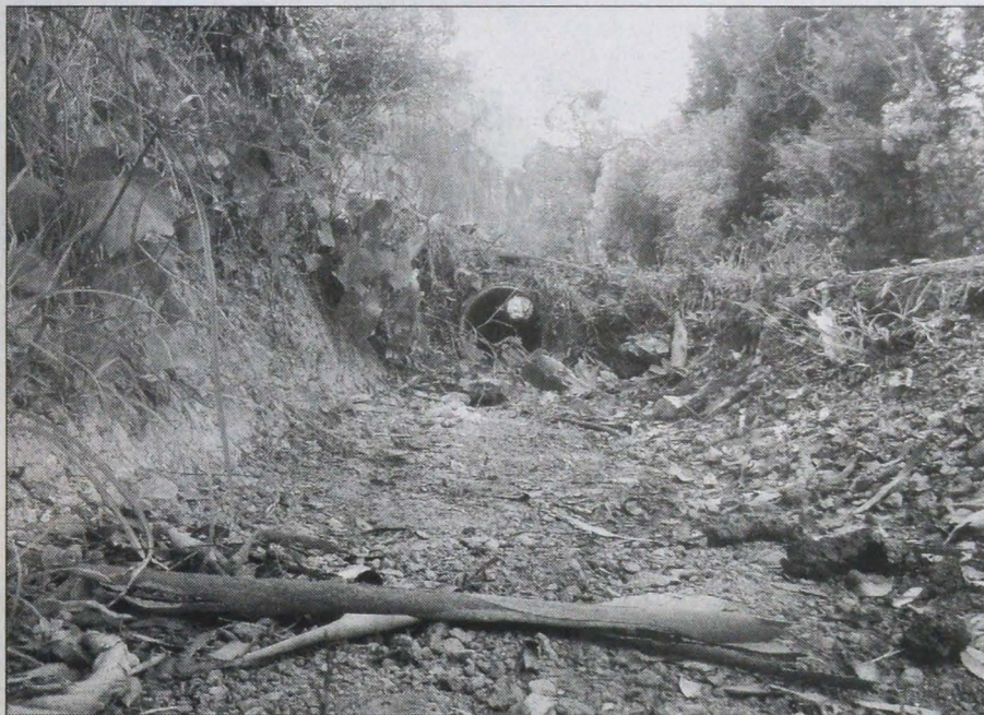
Flood prone: Culvert in Melbourne Hill Road. Note the narrow drainage pipe, which frequently blocks with debris following a downpour. (Picture by Brianna Piazza)
