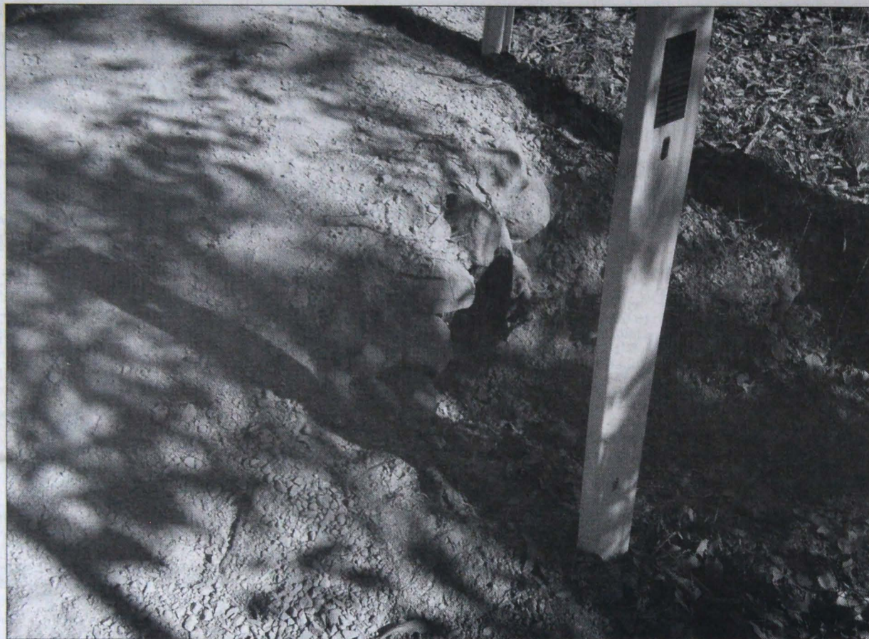
Poor work alleged: 'Rebuilding' this crossing has resulted in this dangerous hole.
